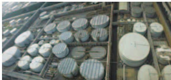
▶ Wastewater Treatment Plant (After improvement)
